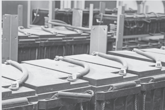
Banks of Batteries Source: iStockphoto/Lee Torrens
